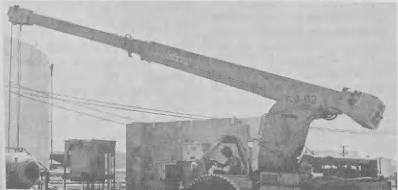
This Pettystone crane with telescope boom is operated by Rene Lamp. Pettystone grua aki cu telescope boom ta ser opera pa Rene Lamp.
